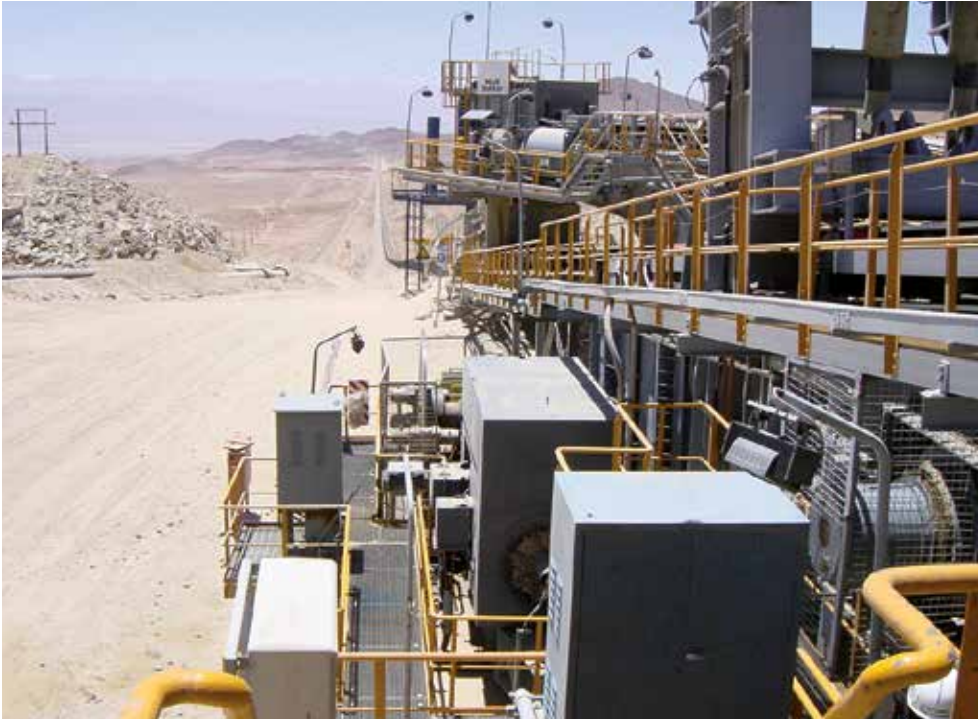
Mining / conveying systems
